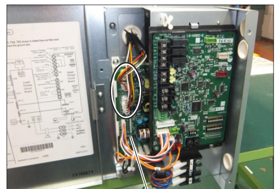
Power circuit board
